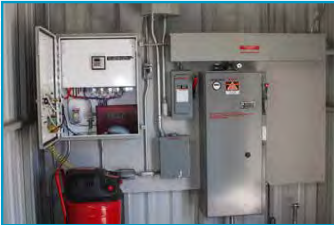
Motor Control Center
