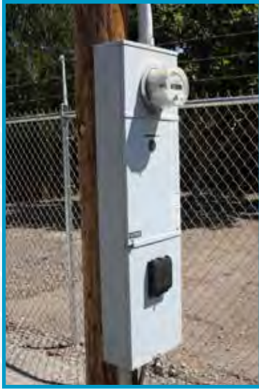
New Electrical Box
