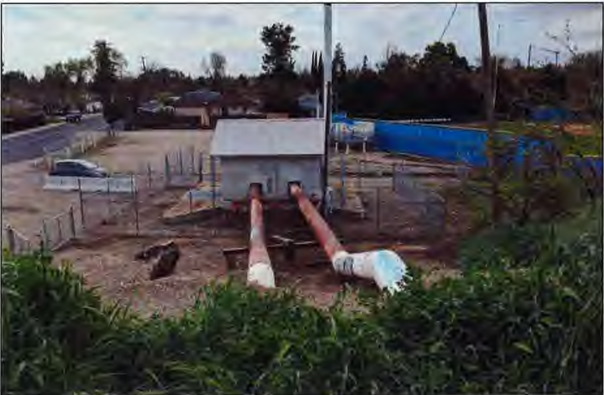
Photograph 4. Wisconsin Pump Station - view to South from top of tributary slough levee
