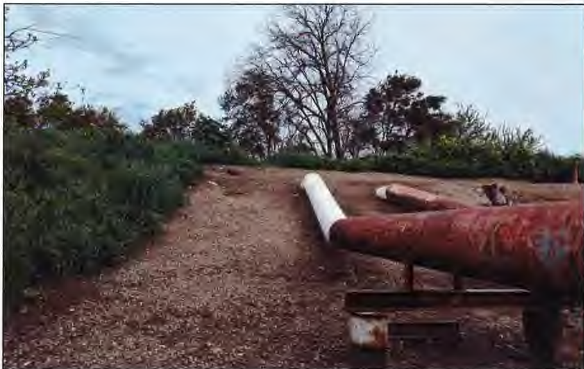
Photograph 2. Wisconsin Pump Station discharge pipes - view to North
