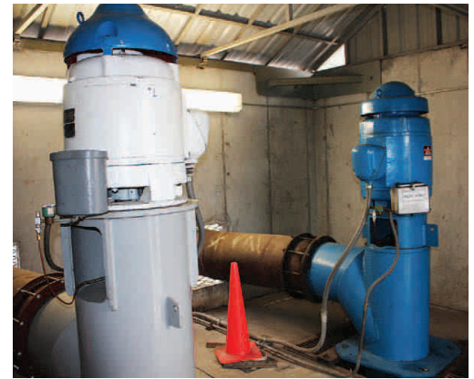
WISCONSIN PUMP STATION
