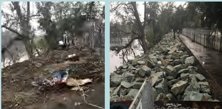
REMOVING RESIDUAL TRASH LEFTOVER FROM THE ILLEGAL CAMPERS AND ROCK PLACEMENT ALONG THE EAST SIDE OF THE PROJECT AREA.
