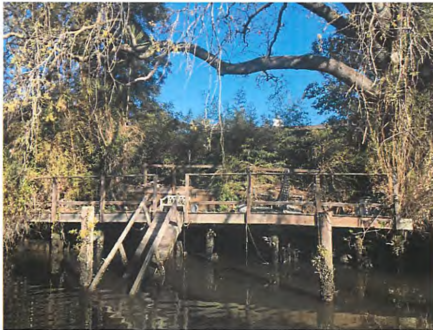
1510 S. W. Tuxedo Ave.: A dilapidated dock has fallen into the canal and dense vegetation overhangs the canal.
