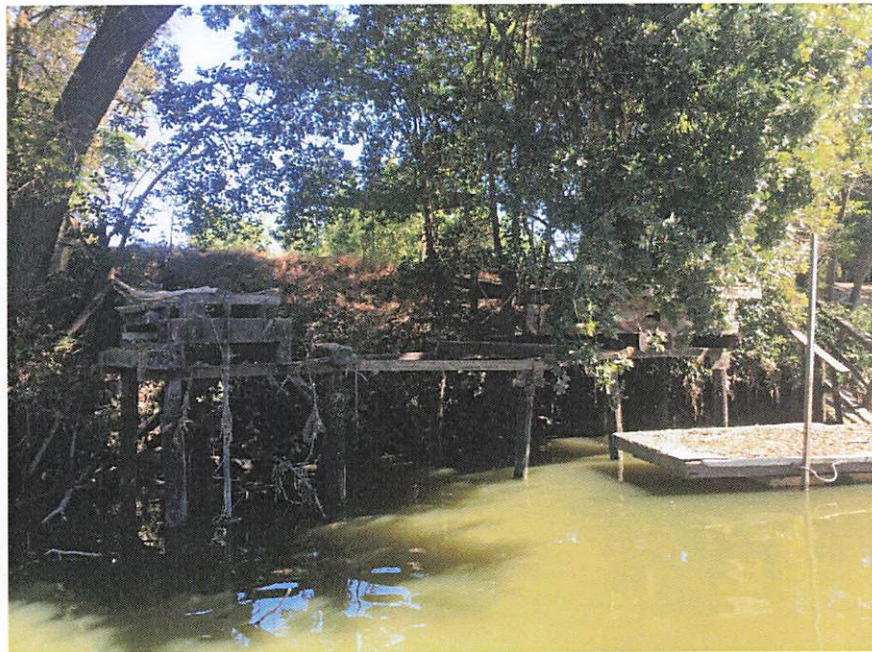
1608 W. S. Tuxedo Ave.: dilapidated pump platforms and a waterside slope ready for riprap.
