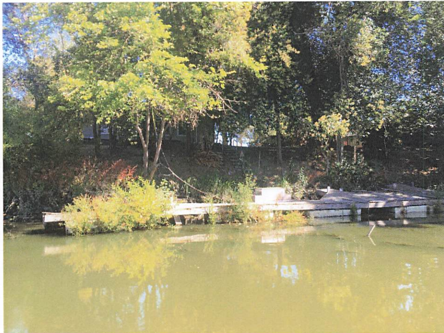
1826 W.S. Tuxedo Ave.: Dilapidated dock and waterside slope bare of vegetation.
