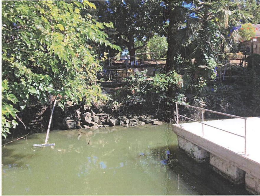
2374 Canal Drive: The homeowner has requested riprap for her levee waterside slope this fiscal year.
