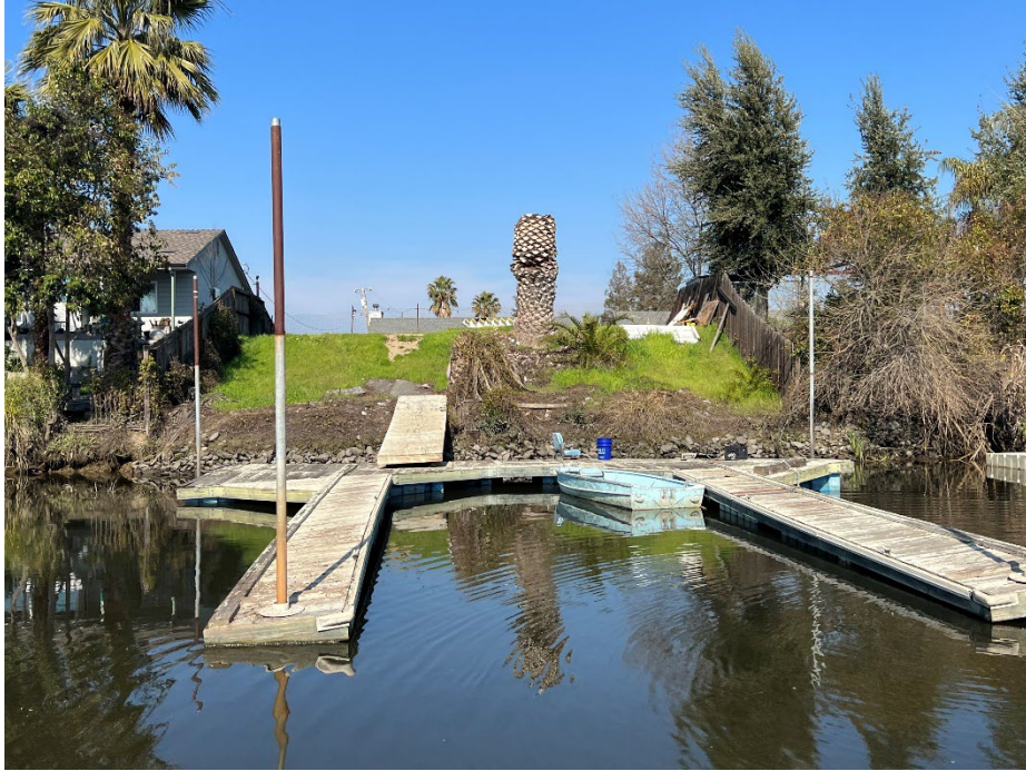
2286 Canal Drive: A good candidate for 18" minus riprap.
