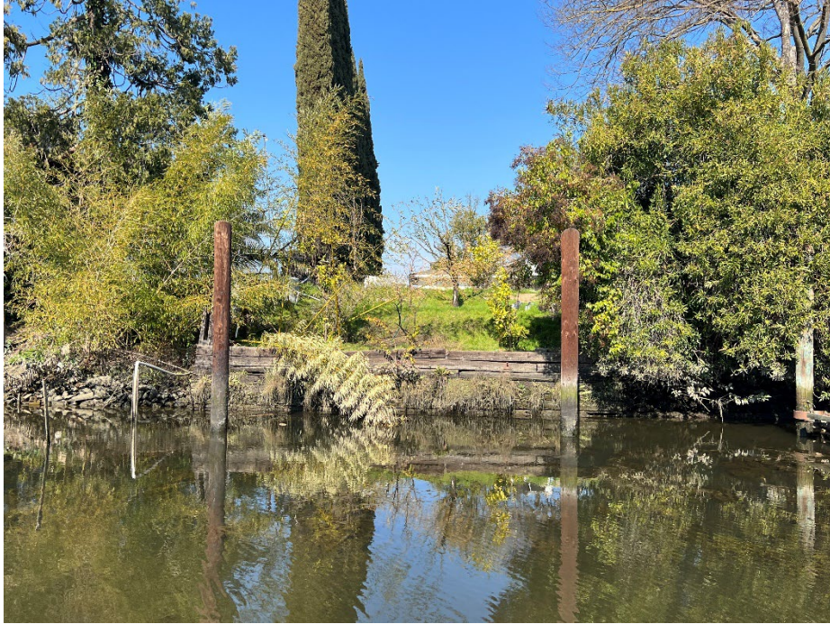
2038 Canal Drive: A good candidate for 18" minus riprap.
