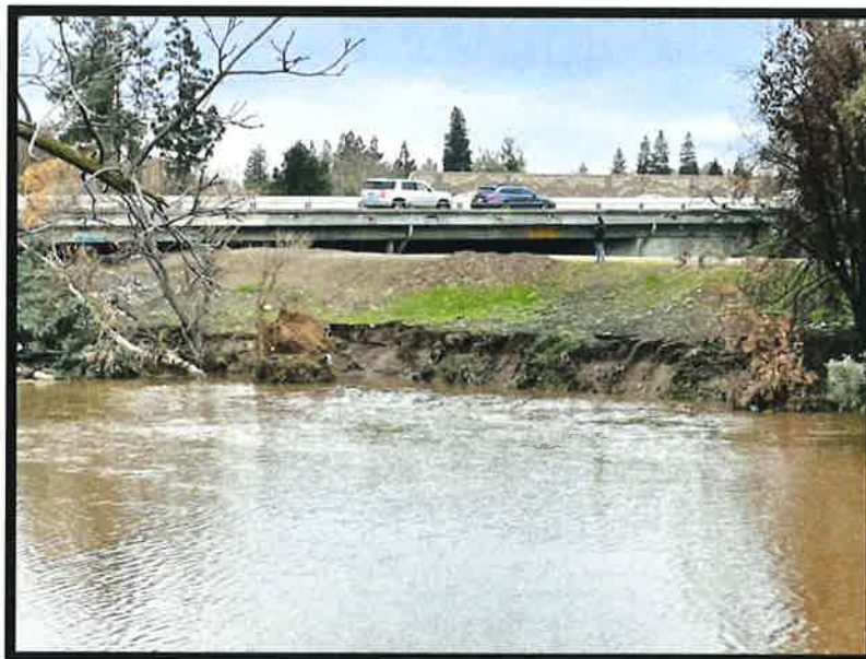
Calaveras River Levee Damage - January 2023
