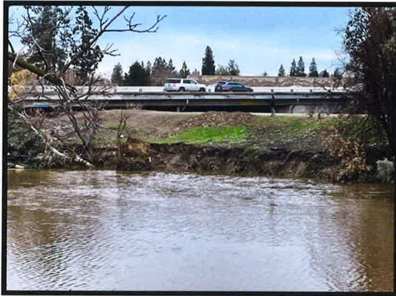
Calaveras River Levee Damage - January 2023
