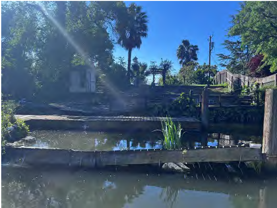
1641 Walnut St.: Dilapidated docks and decking.
