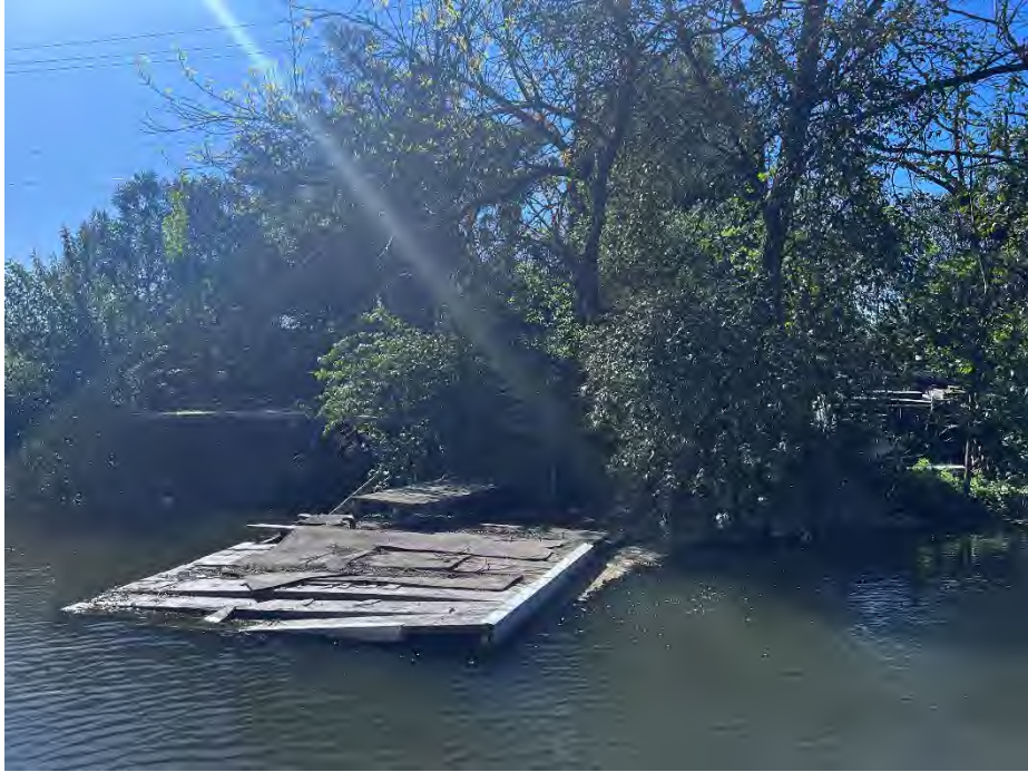
1852 Shimizu Dr.: Dilapidated dock and debris piles litter the waterside slope beneath dense vegetation.
