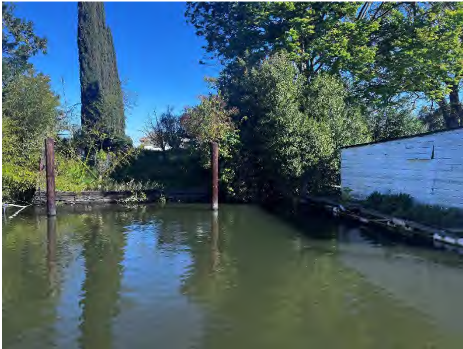
2038 Canal Drive: Dock remnants in channel (spuds) and dense vegetation on waterside slope.
