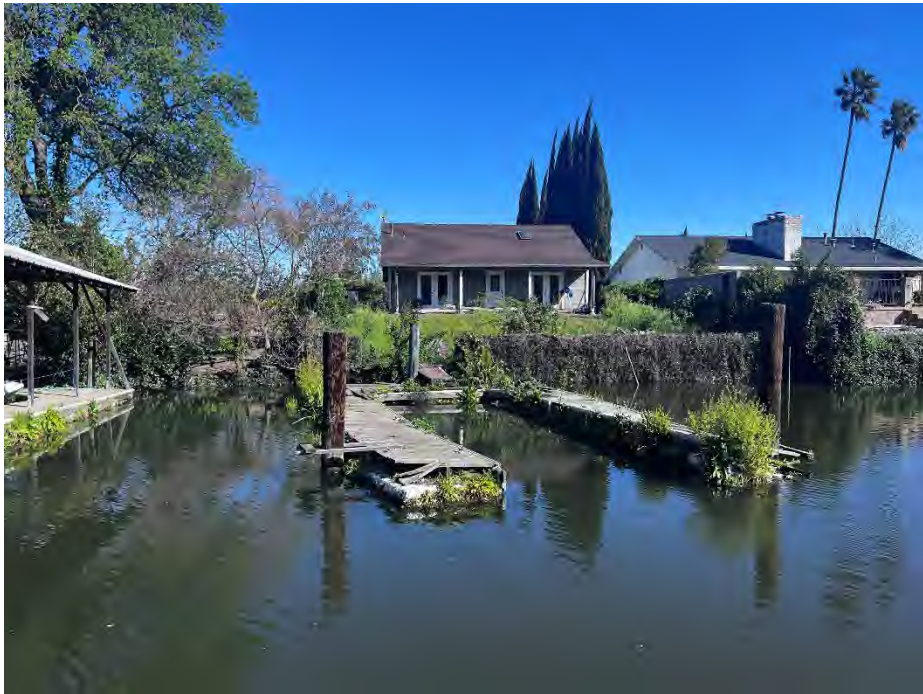
2364 Canal Drive: Decaying dock in water and no rock on waterside slope.
