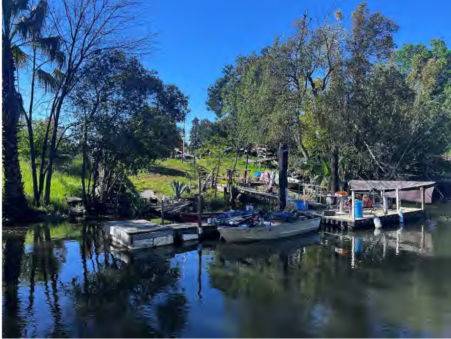
1625 Walnut St.: Dilapidated docks, piles of debris and no rock on waterside slope.
