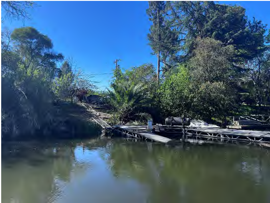
1535 Walnut St.: Overgrown brush, dock in state of disrepair and debris piles on waterside slope.
