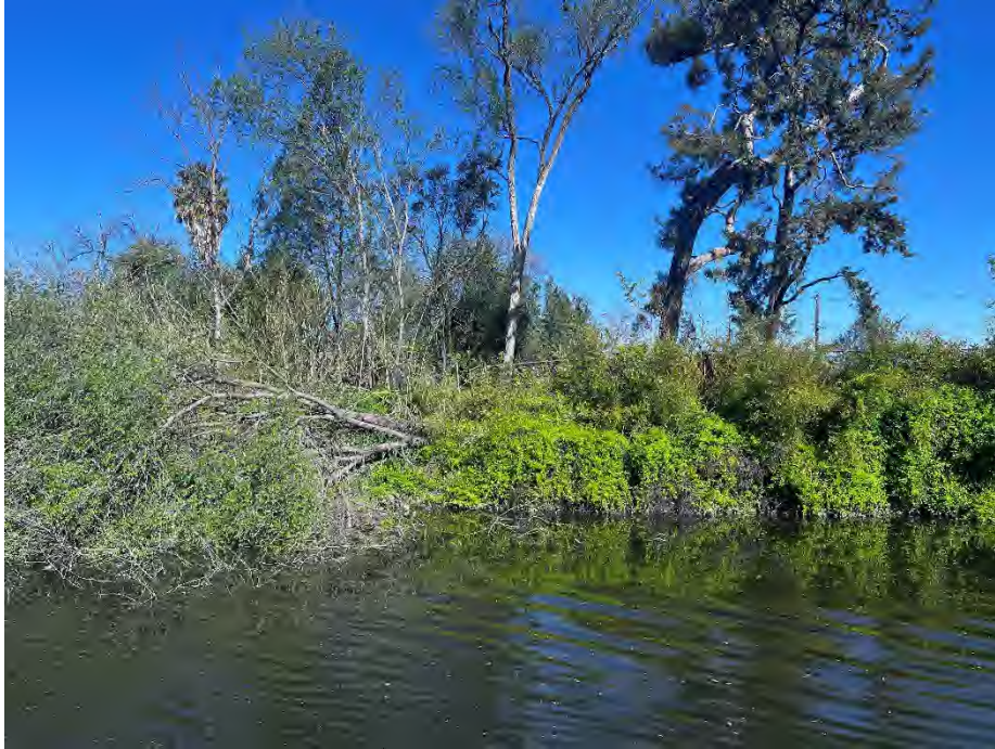
1842 W.S. Tuxedo Ave.: Tree felled by the recent high wind events. This area needs further inspection to determine extent of damage to levee slope, if any.
