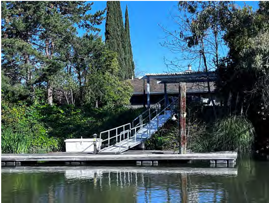
3028 Canal Drive: No rock on waterside slope.
