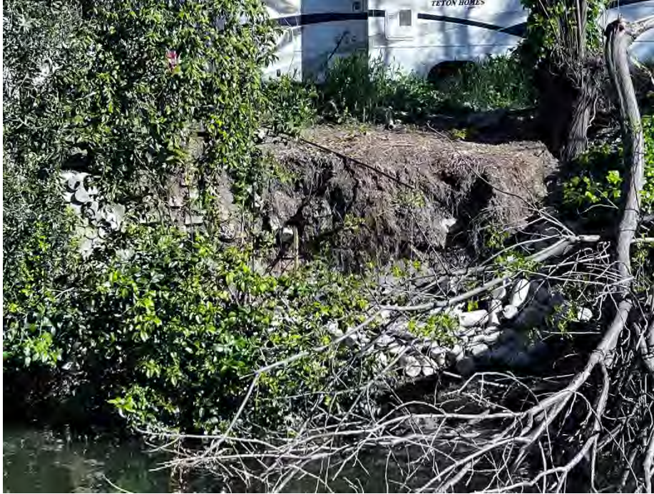
2121 Fontana Ave.: A portion of the concrete cylinder 'headwall' collapsed into the water.
