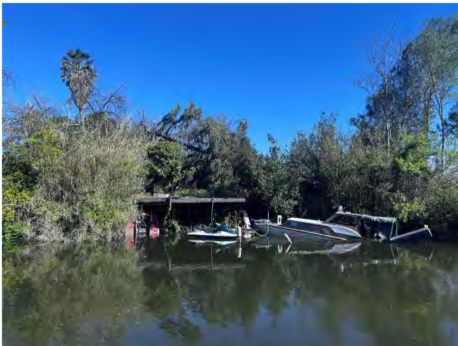
1848 W.S. Tuxedo Ave.: This house is scheduled to be demolished by the City of Stockton this year. Note the tree that fell through the roof and the sunken boat – it has current registration (right, foreground).
