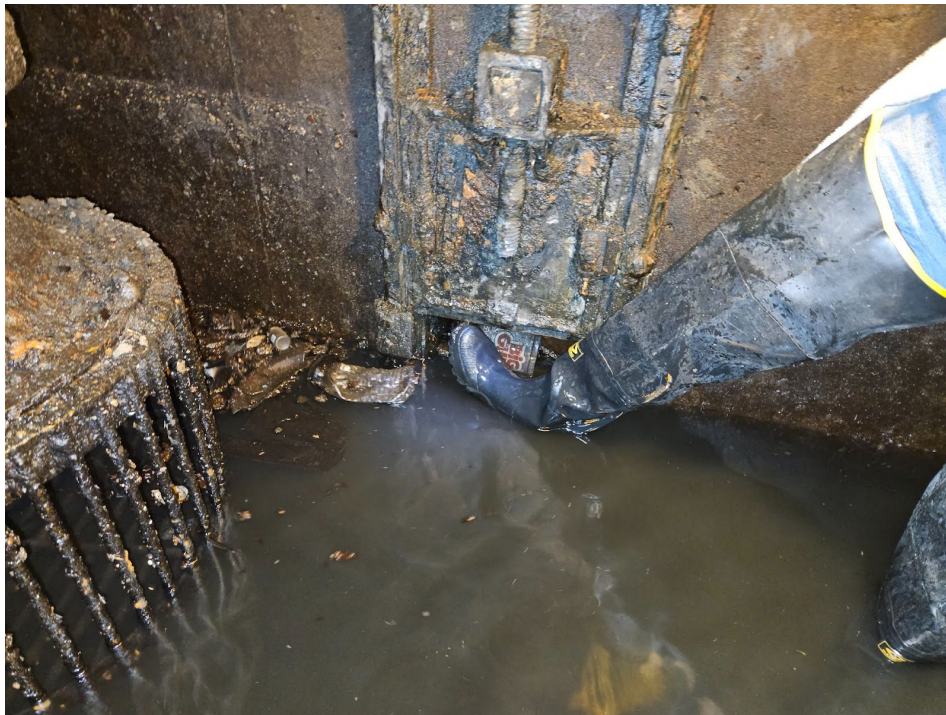
Gate opened half way- Extreme corrosion- workers boot for size reference
