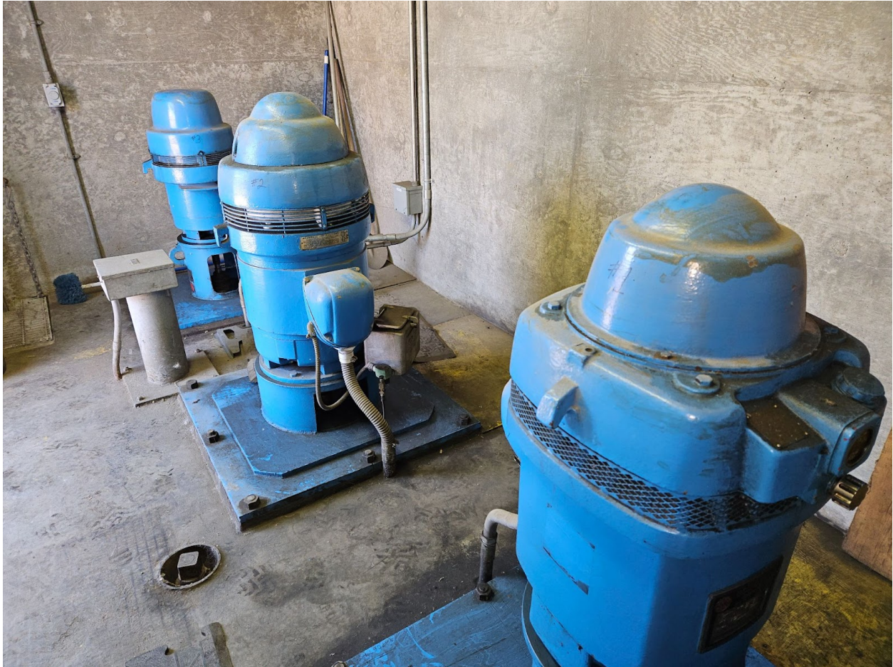
The gate operator nut can be seen on the floor - In between pumps (1) and (2 & 3)
