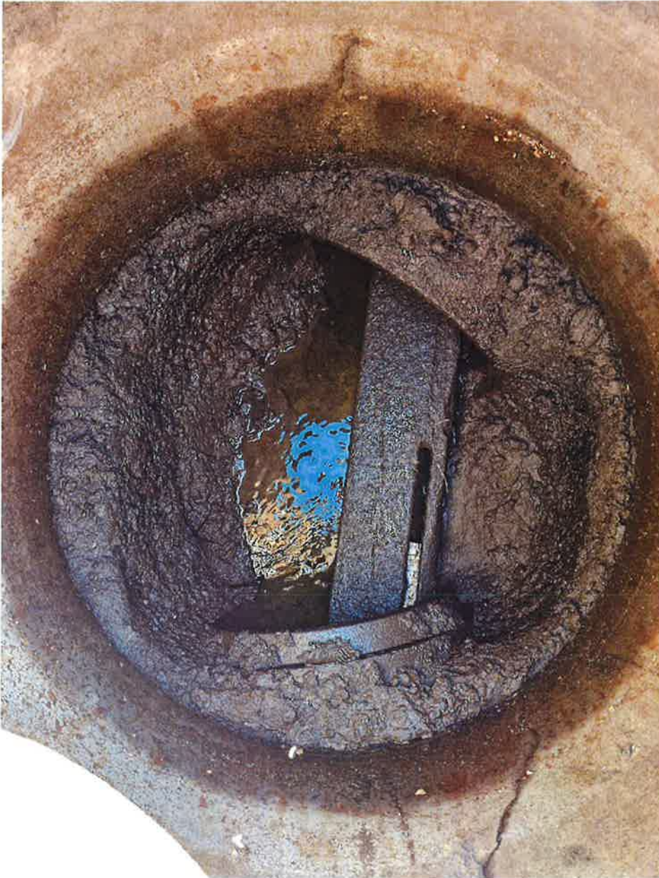
MH-3 Figure 5: Condition of MH-3. A lodged 2x6 piece wood debris shown.
