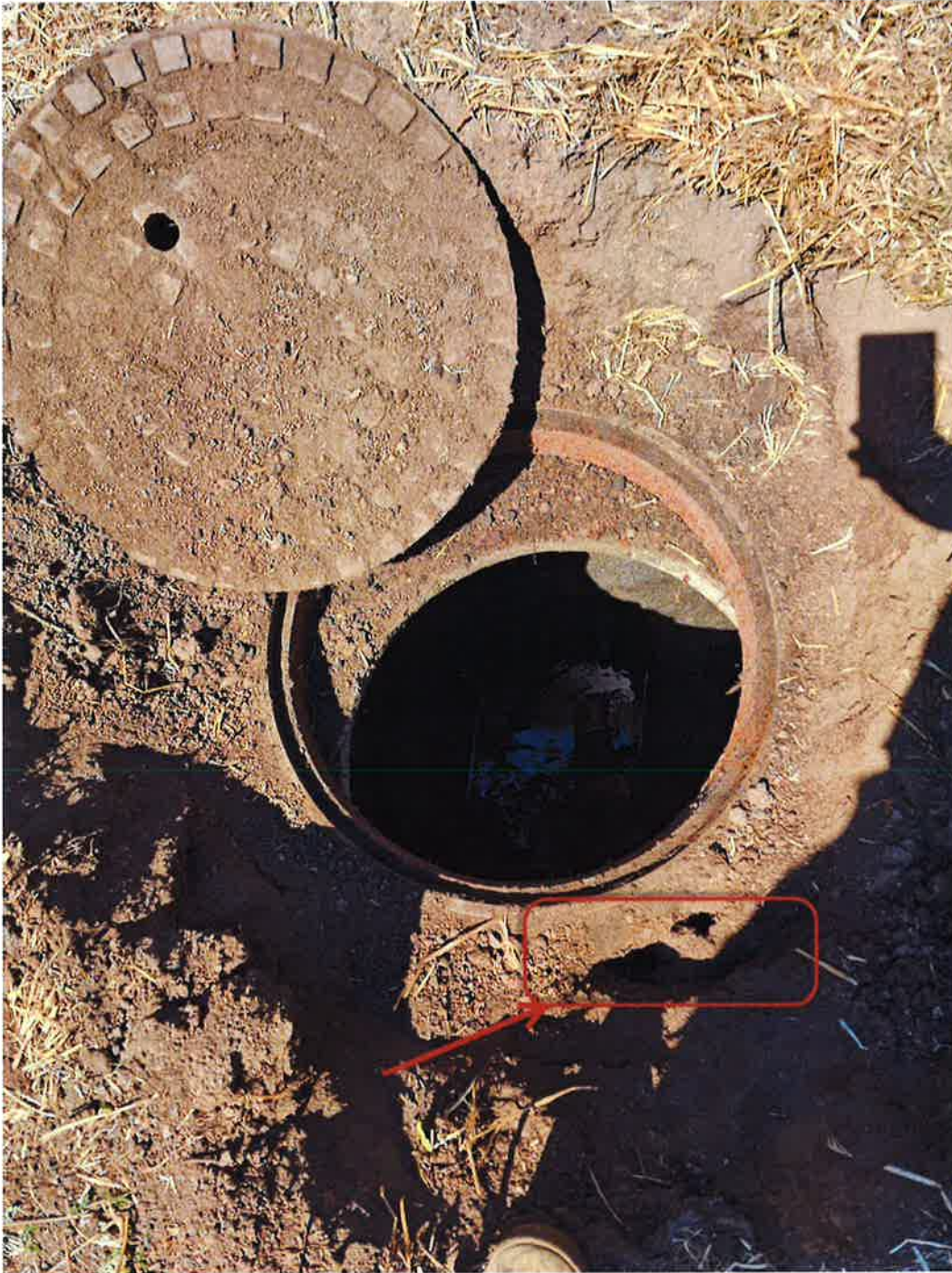
MH-1 Figure 4: Condition of MH-1; misaligned lid/rim allowing debris to fall in.
