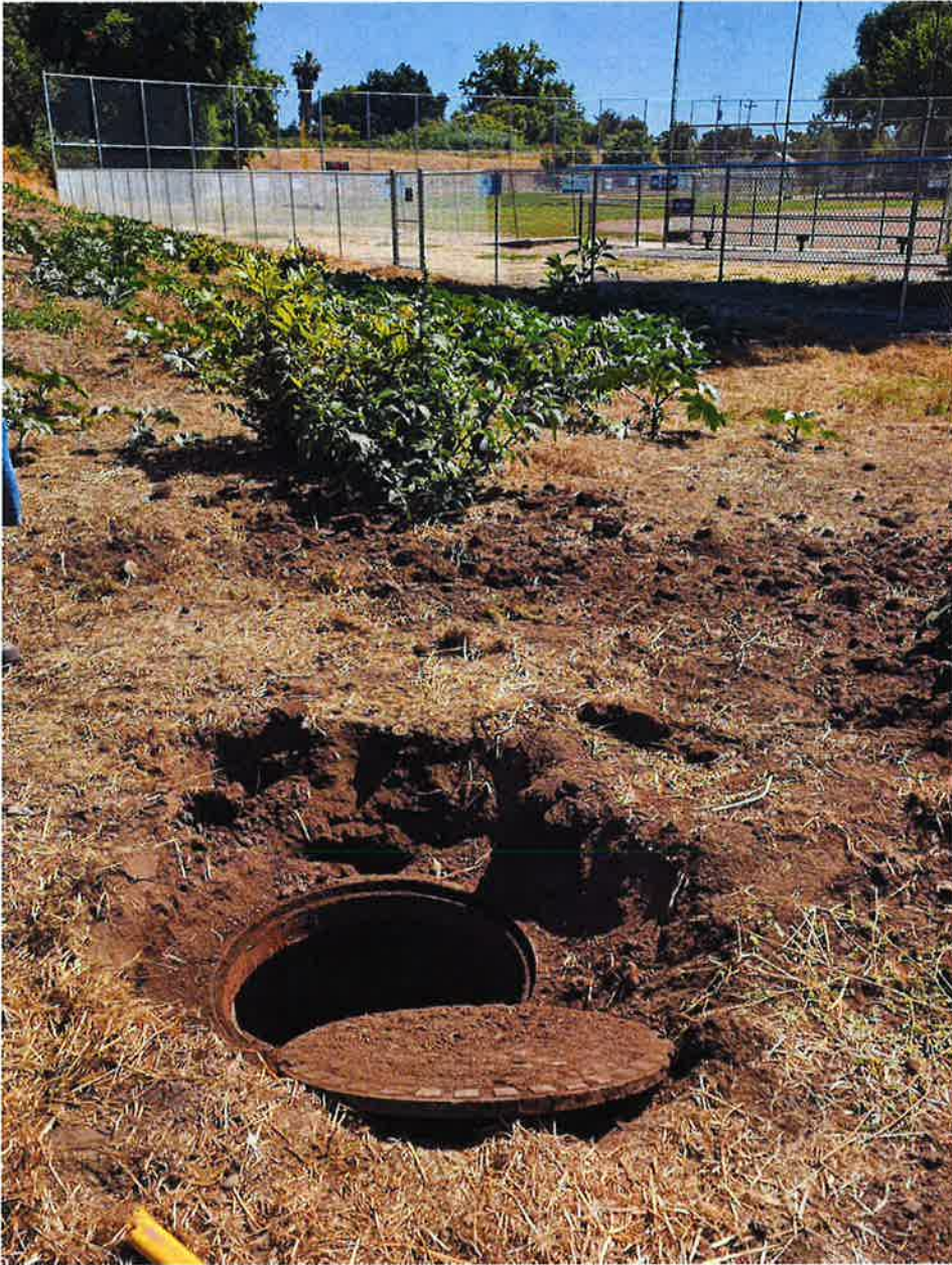
MH-1 Figure 3: Condition of MH-1 buried approximately 14-inches. Recommend regrading or extending rim/lid.
