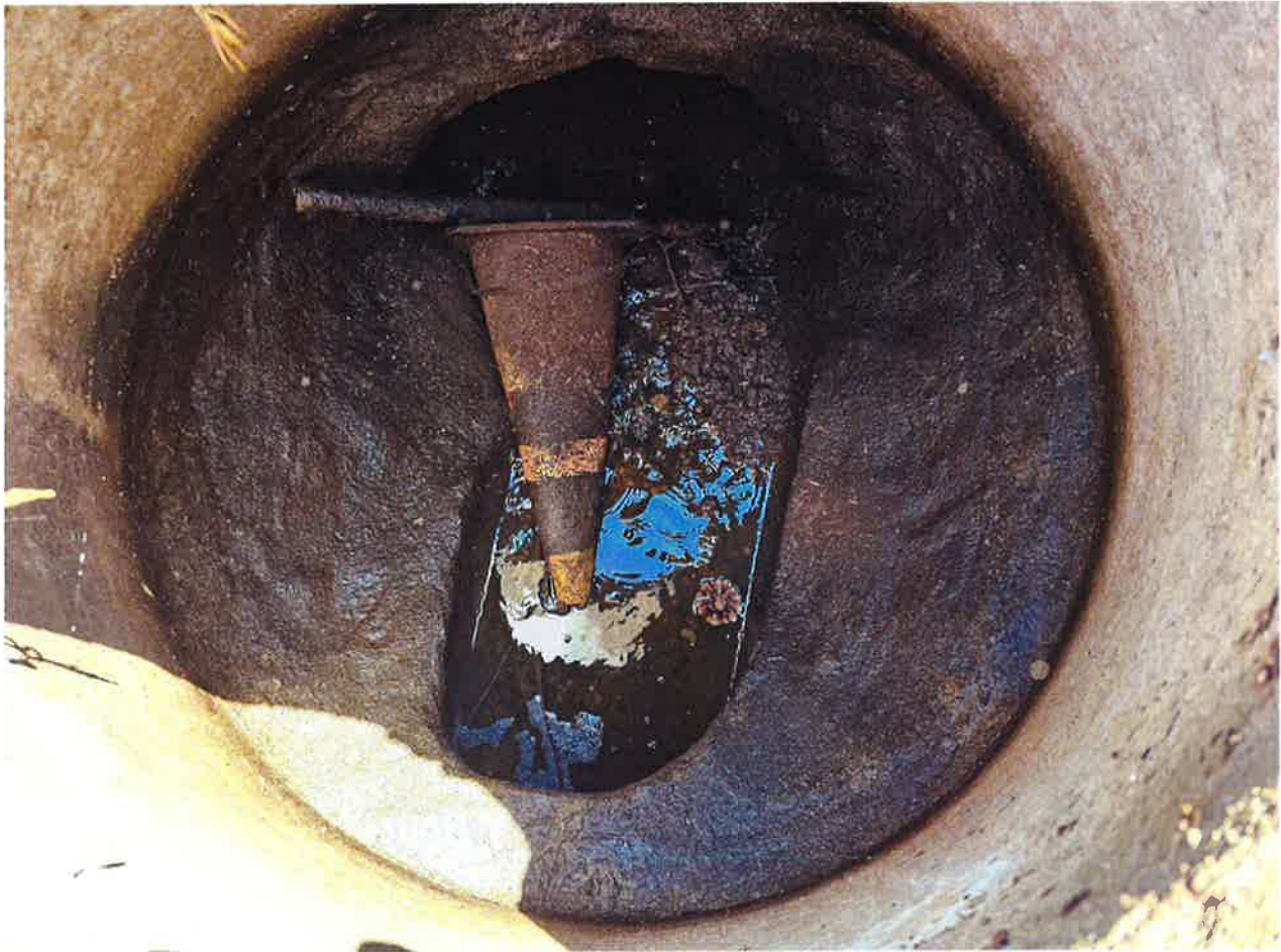
MH-1 Figure 6: Condition of MH-1 approximately 6 feet deep.
