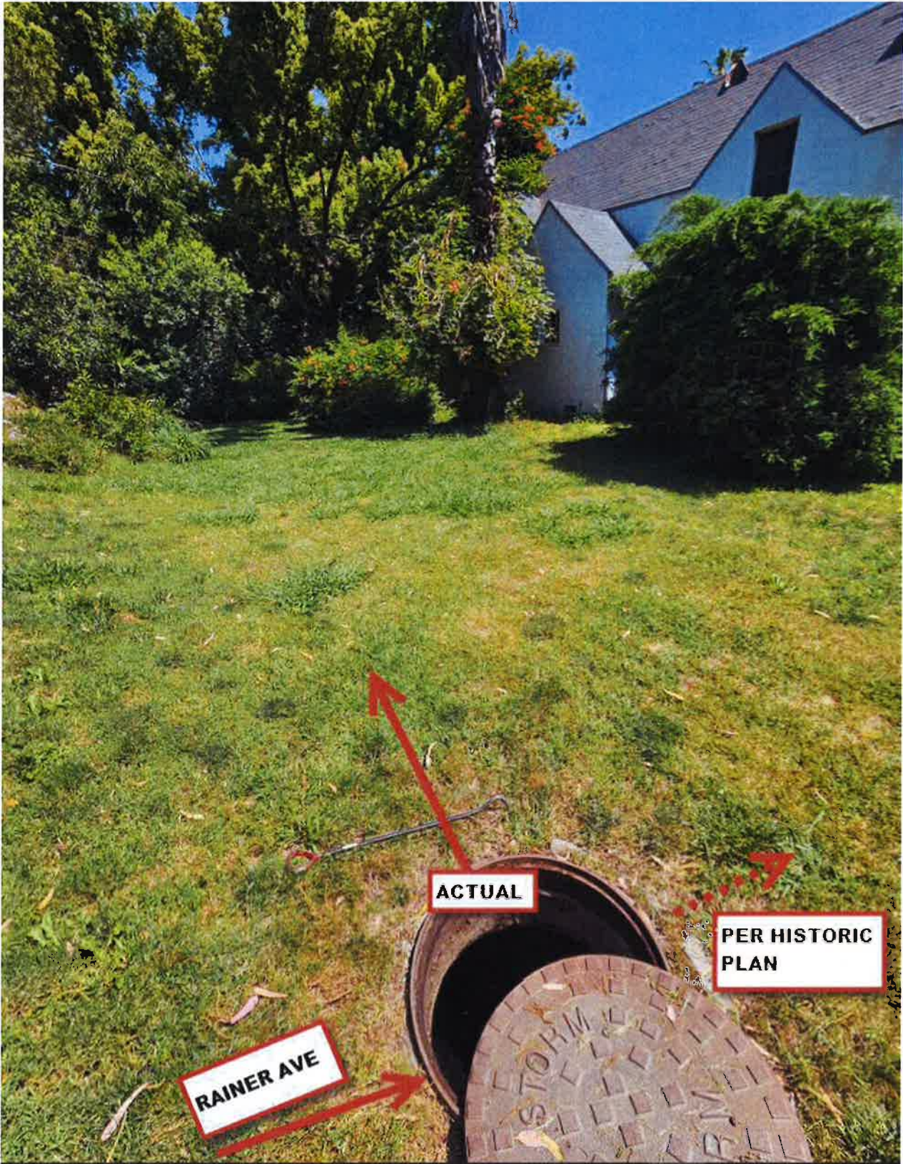
MH-0 Figure 3: Condition of MH-0; 90 degree turn vs plan showing straight.
