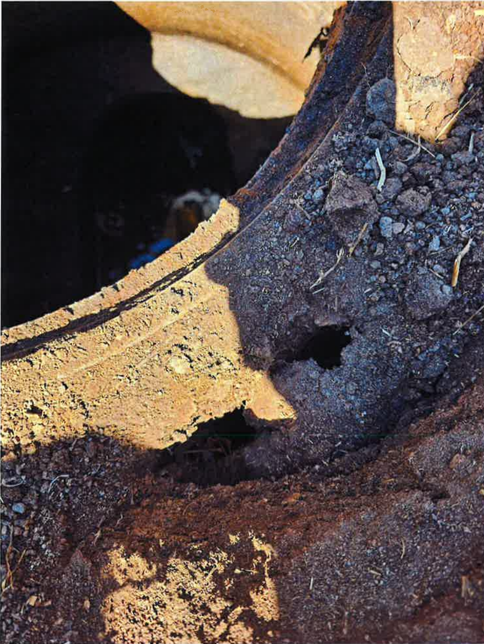
MH-1 Figure 5: Condition of MH-1; misaligned lid/rim allowing debris to fall in.
