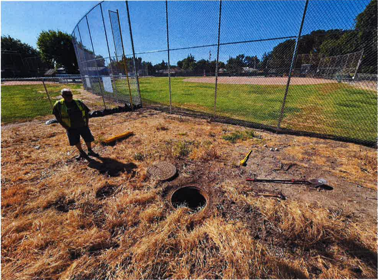
MH-3 Figure 3: Condition of MH-3 buried approximately 2-inches located outside of Hoover-Tyler baseball fields and fencing.
