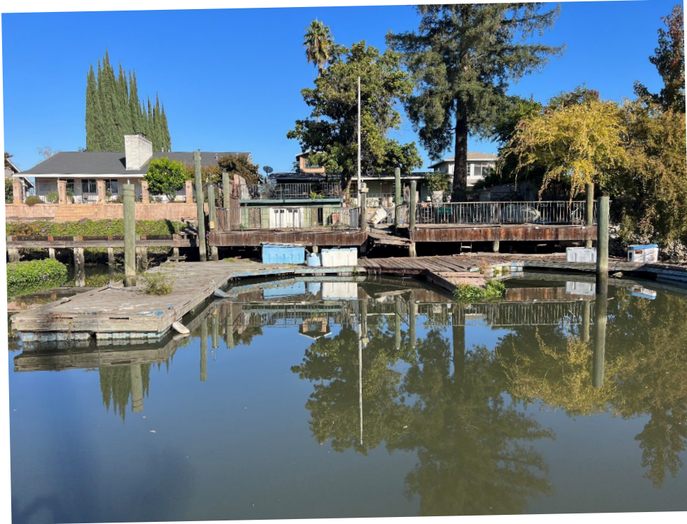
2344 Canal Dr.: The property owner here decided they wanted RSP, but are not willing to remove the dilapidated dock or deck.
