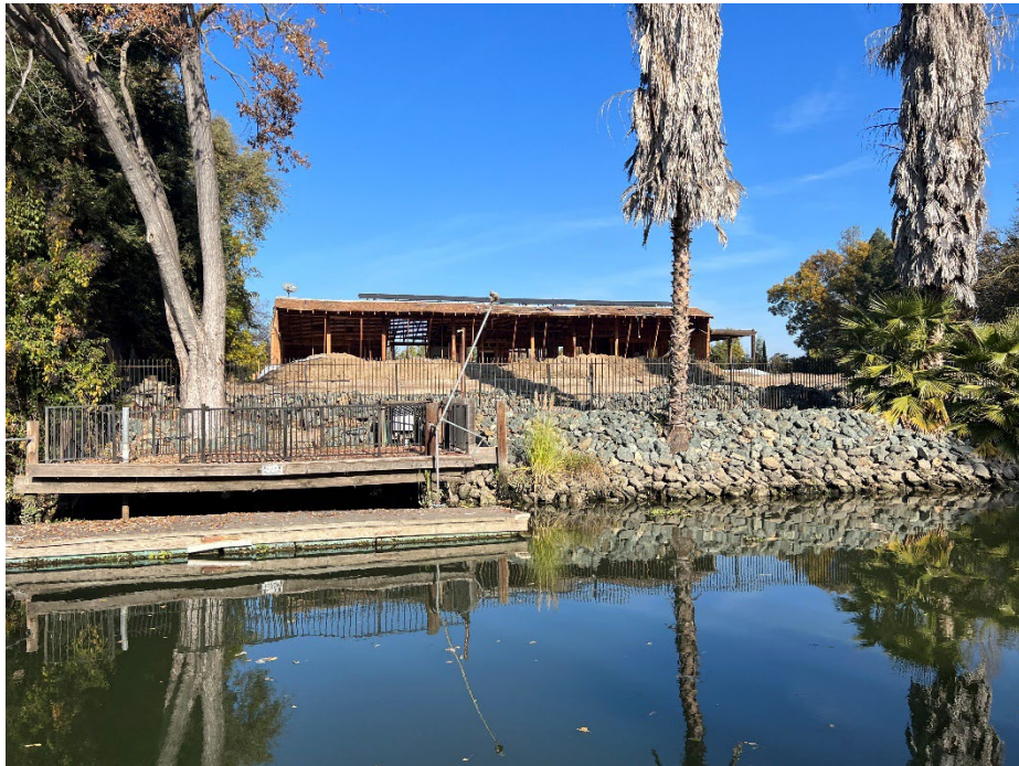
3216 Moering Ct.: Piles of soil sit atop the levee crown.
