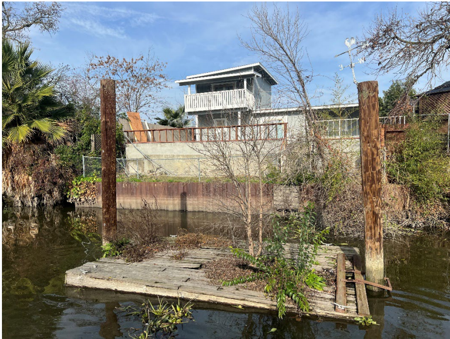
1522 S Tuxedo Ave.: Grading of the levee crown was spotted at this property during the last inspection. Now a retaining wall raise and new house paint are obvious.
