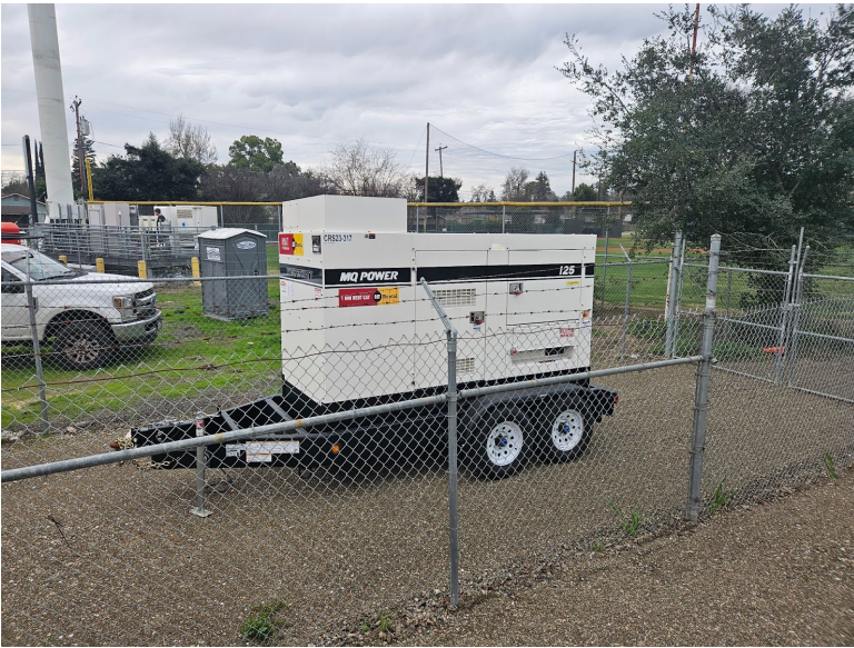
125 KW - Gen set placed at Wisconsin Pump Station for emergency response.
