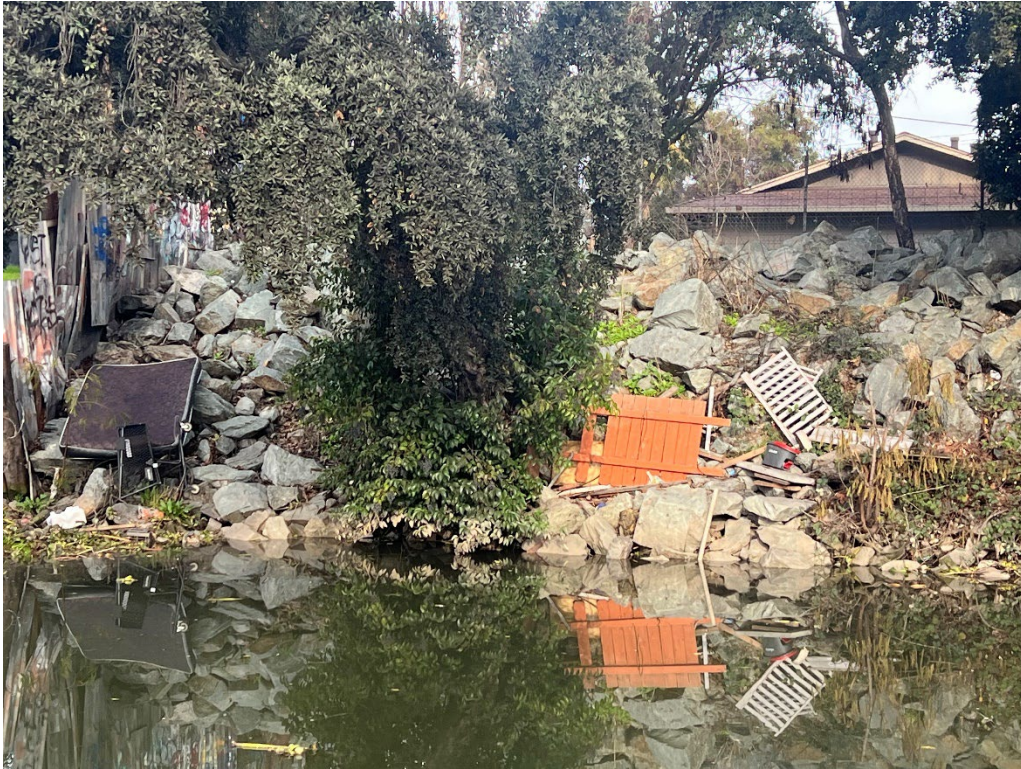
Debris continues to build up at the terminus of the sidewalk east of Fontana Ave.
