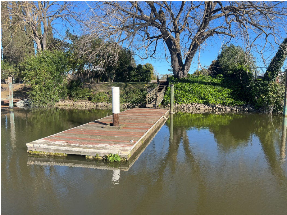
2026 Canal Drive: RSP would look good on this slope.
