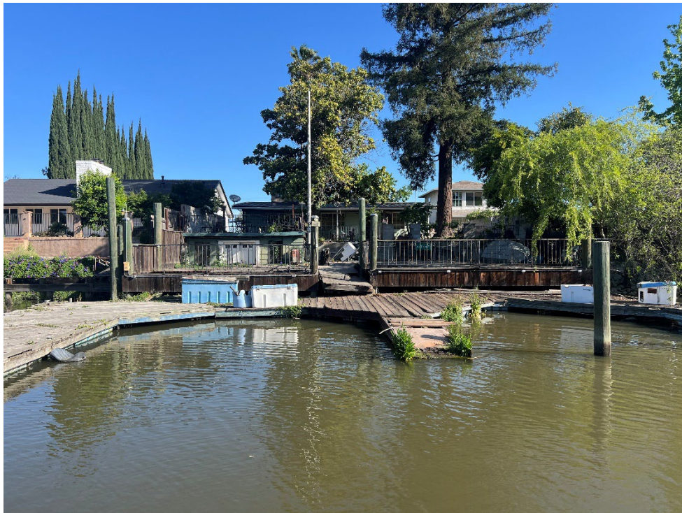
2344 Canal Drive: This property owner requested RSP, but hasn't seen his waterside levee slope in his entire life. He also wants the District to remove all of the dilapidated wood decking.
