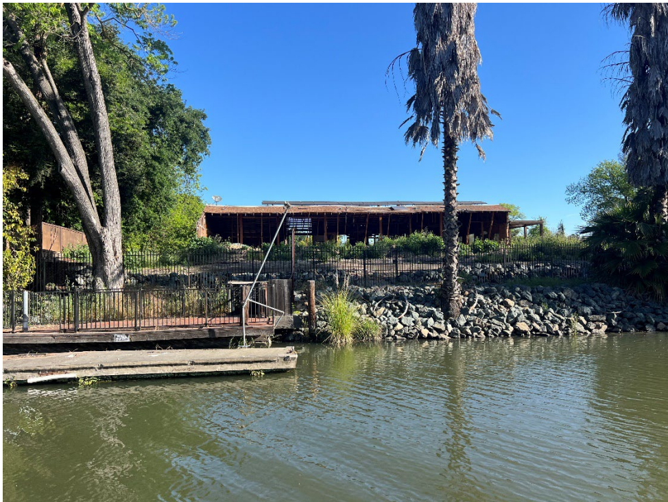
3216 Moering Ct.: The house remains gutted, with no evidence of new work in a couple of months.
