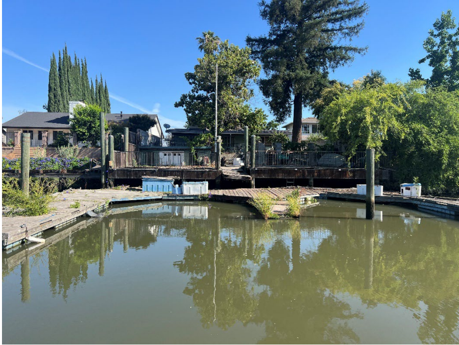
2344 Canal Drive: The property owner expressed interest in RSP and in having the District remove the dilapidated deck, dock and everything on the slope that would preclude him from receiving RSP.
