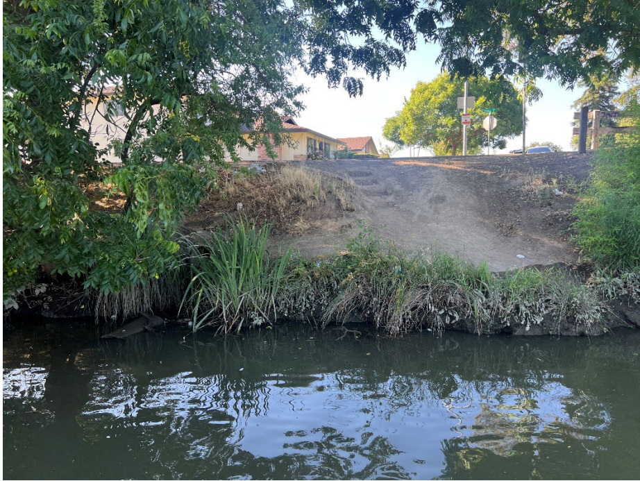
Sta. 81+00 (Occidental Ave. & Shimizu Dr.): A neighbor across Smith Canal pointed out that the City of Stockton's storm drain did not have a flap gate on it (in photo, left of the dirt area).
