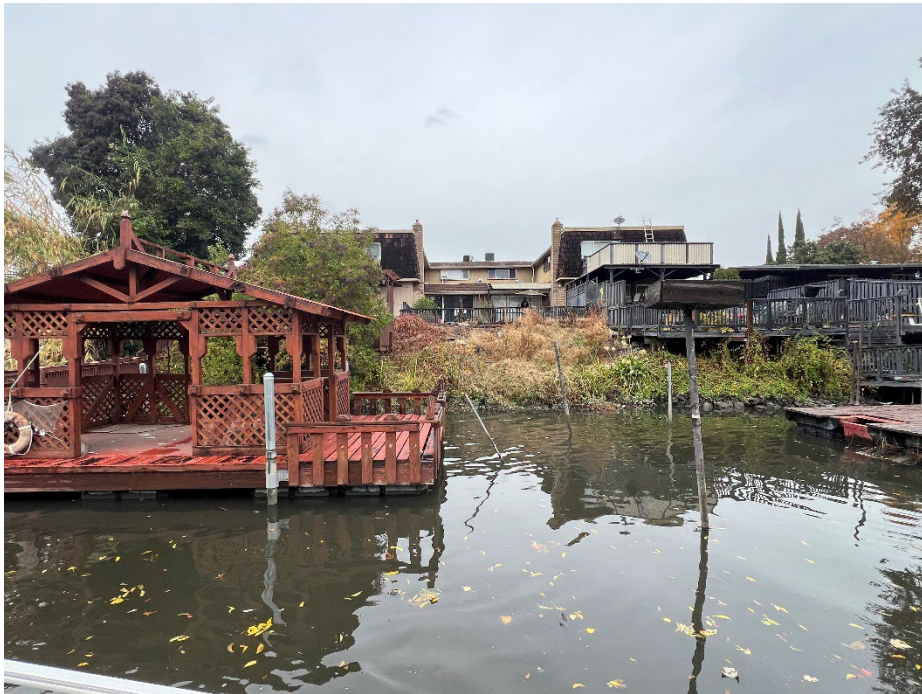
2008 Grange Ave.: RSP was placed along the waterside slope nearly two decades ago but appears to have slipped into the canal over time.
