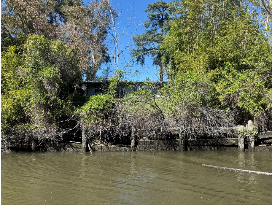
1466 S. Tuxedo Ave: Undercut on property appeared to be excessive erosion but unable to contact property owner.
