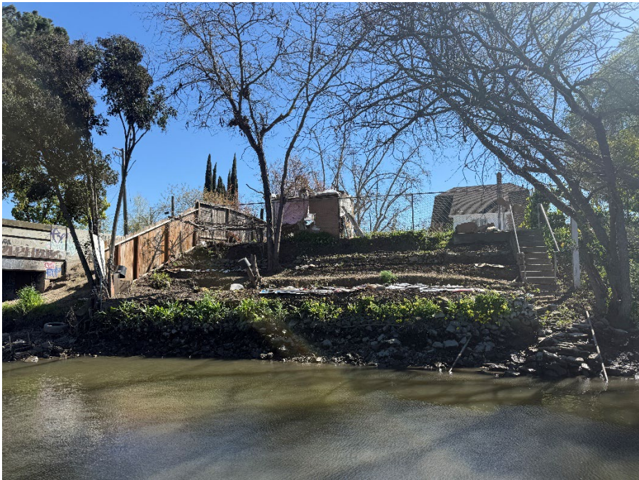
Property adjacent to Pershing Ave: No repairs to the waterside slope have yet occurred.
