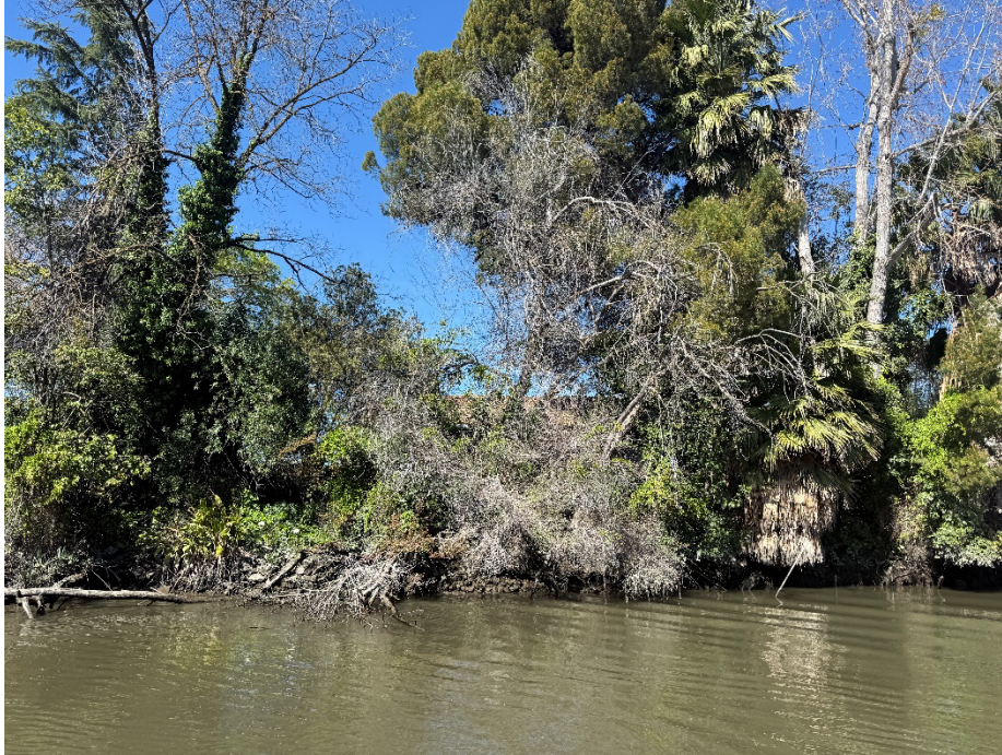
2004 Canal Drive: A property that had RSP placed in past years but had a slip occur over the winter months.
