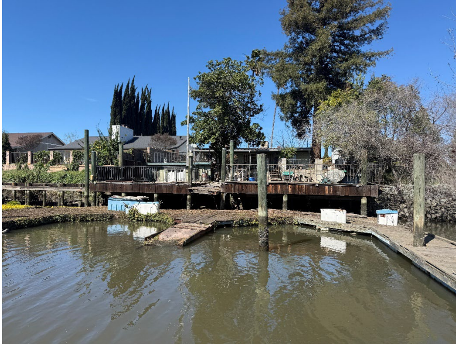
2344 Canal Drive: Property owner initially wanted RSP, then refused it, then decided he wanted the District to provide him with 3" rock.
