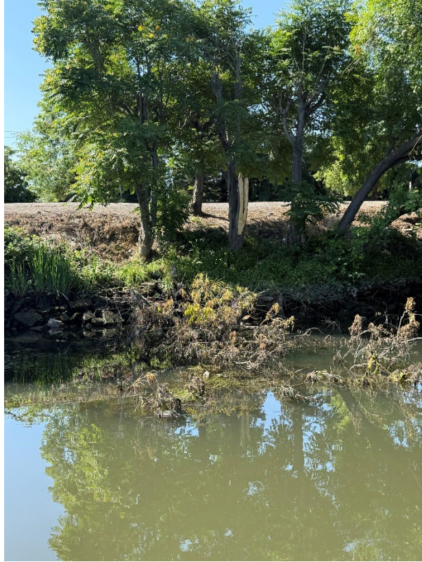
Sta. 55+70: Another fallen tree in water.
