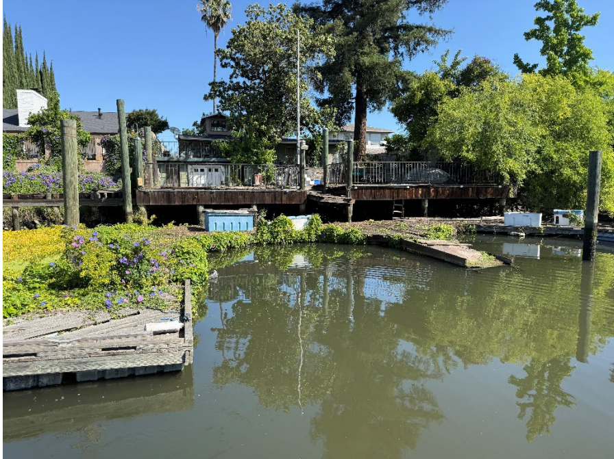
2344 Canal Drive: Property owner originally requested RSP and requested his dilapidated dock and appurtenances be removed a few years ago but was denied due to the unavailability of funds. Currently, the owner wants to keep his dock in place and the District to supply him 1-inch rock for unspecified use.
