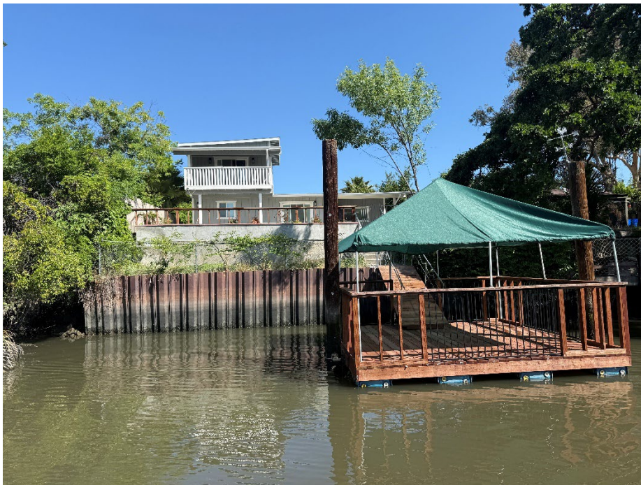
1522 S. Tuxedo Ave: Property owner constructed a pool on top of the levee crown several years ago (see Google Earth screen shot next photo).
