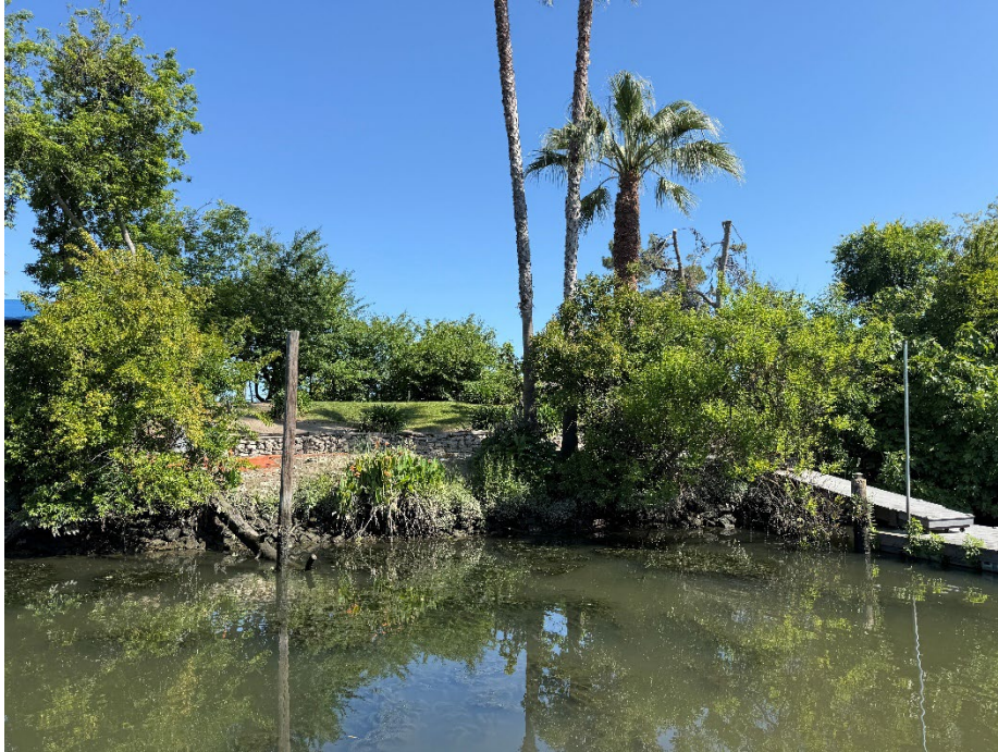
2072 Canal Dr: Property owner originally agreed to receive RSP but later reneged due to inconvenience to him because he had a broken leg at the time the rock was to be placed.
