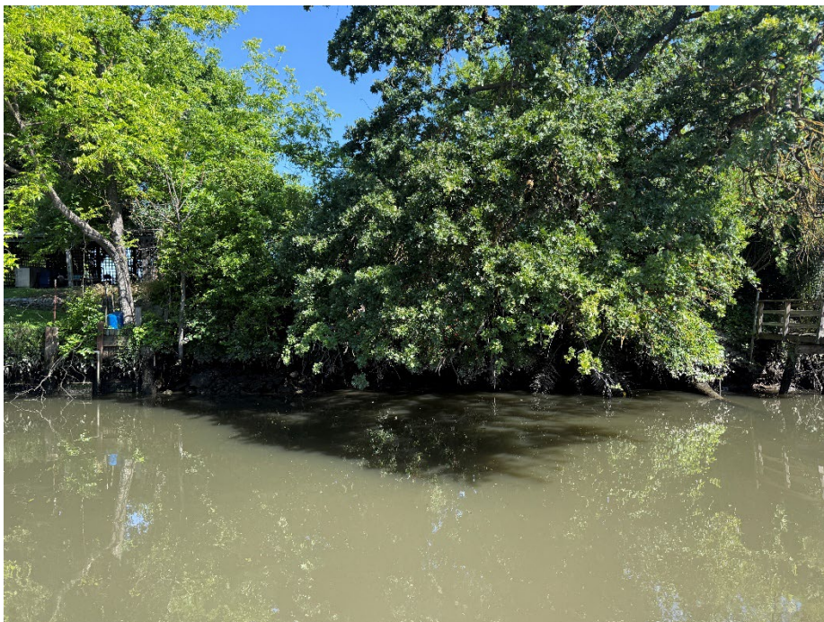
1534 S. Tuxedo Ave: Undercut toe on waterside slope with no visible RSP. The property owner has not contacted the District following brochures and business cards left on house door over the years regarding RSP work.
