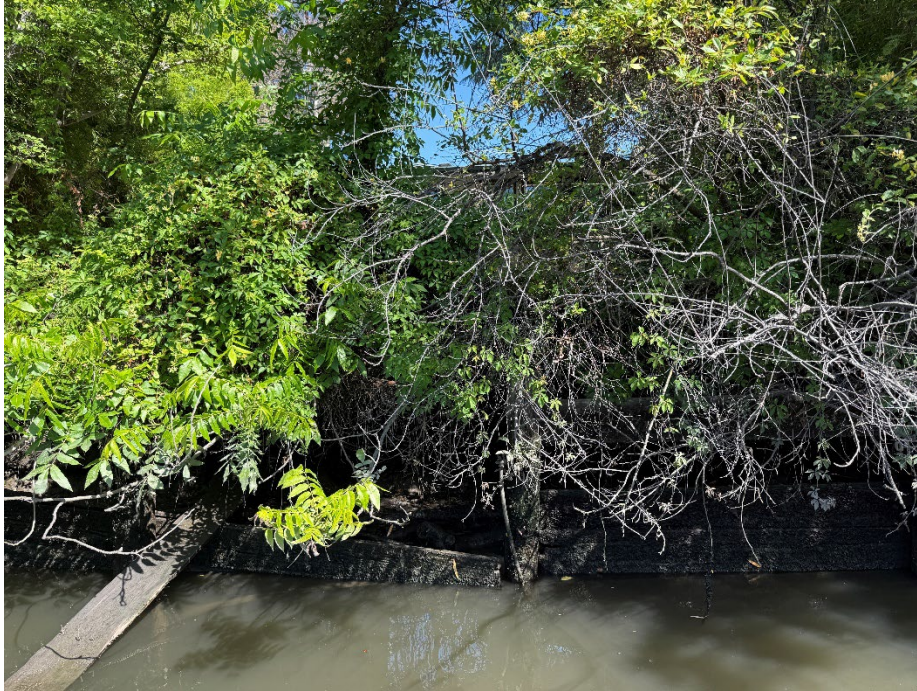
1466 S. Tuxedo Ave: Collapsed wooden headwall at waterside toe reveals eroded bank behind.
