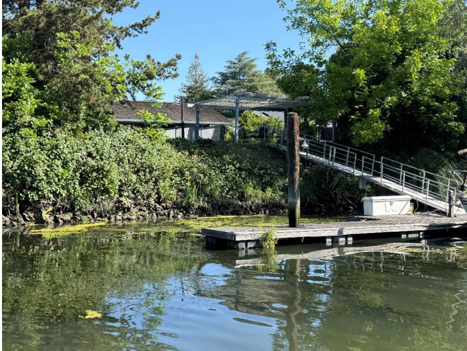
3028 Canal Dr: This property appears to have old RSP on its waterside levee slope.
