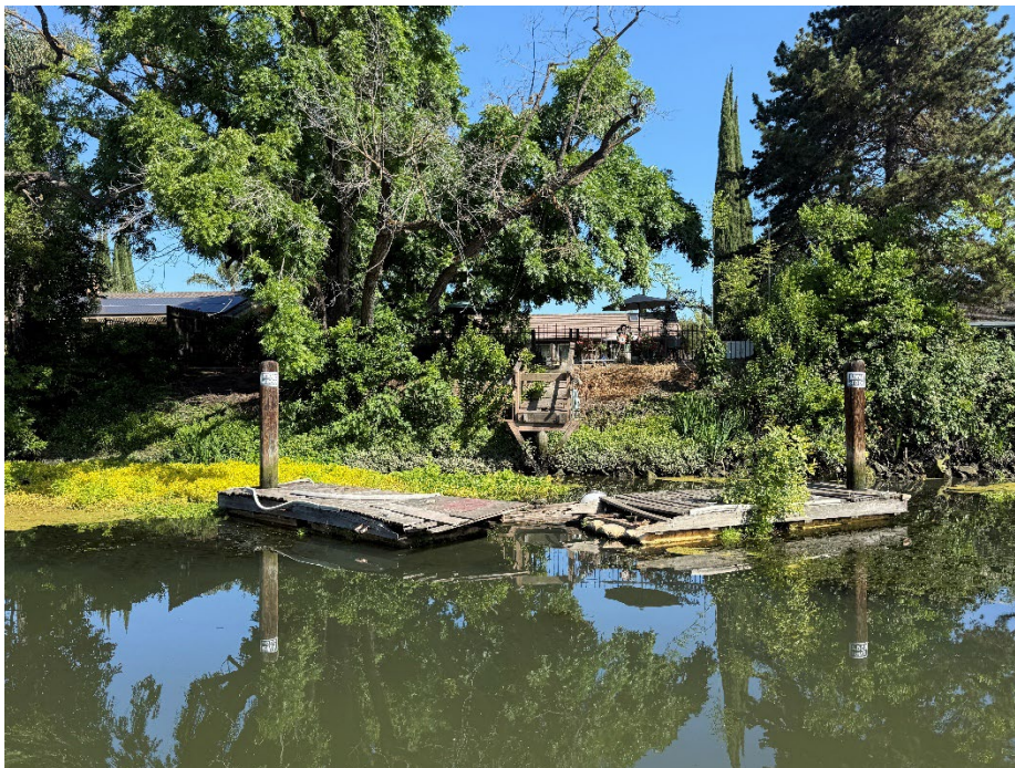
3042 Canal Dr: The last of the properties west of I-5 that has no RSP and has to capability to receive it.
