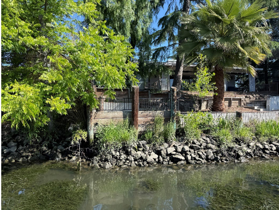
2010 Franklin Ave: A small amount of erosion has eaten away at the property's southwest corner.
