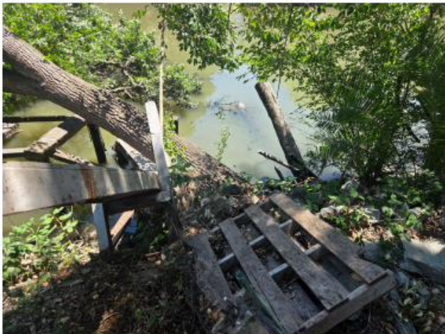
Downed Tree -1608 South Tuxedo
